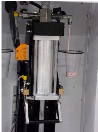
Figure 14: Bleeding the Valve
